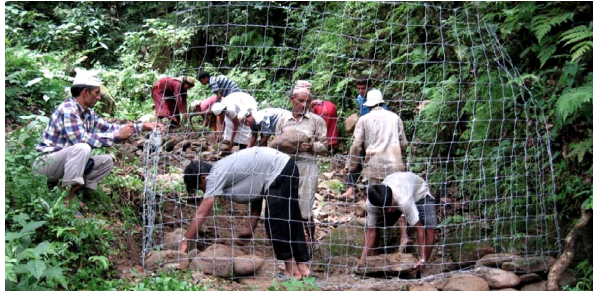
Figure 4. Gabion box filling, one of the activities supported by the Cooperative and carried out by upstream communities in order to decrease sedimentation in the lake and stabilize landslides. Source: LI-BIRD, 2009
